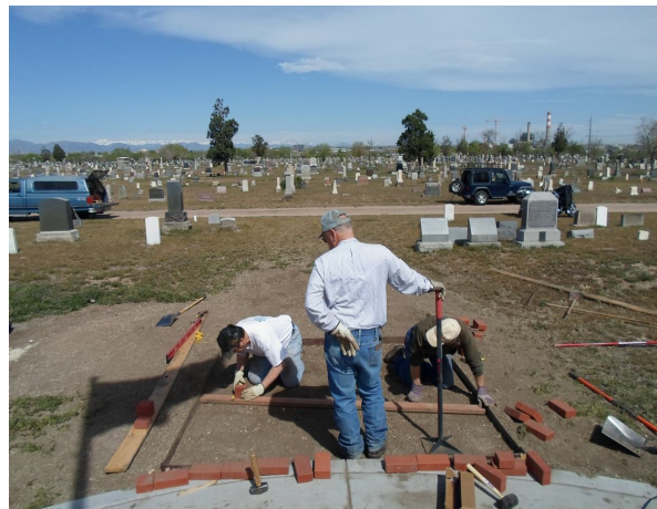
Br. Art Goguen, CC Gene Cheney and PCC Craig Ayler laying the framework for the walkway.
